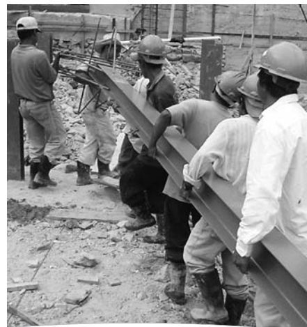
La Esperanza Hydroelectricity project, Honduras
