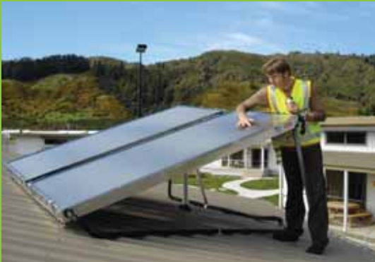
Energy Manager Cees Ebskamp examines solar panels at Rimutaka Prison. Image courtesy of the Department of Corrections.
