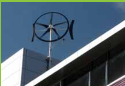
Rooftop-mounted micro wind turbine. Image courtesy of Vector Limited.
