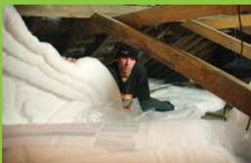
Ceiling insulation. Image courtesy of EECA.
