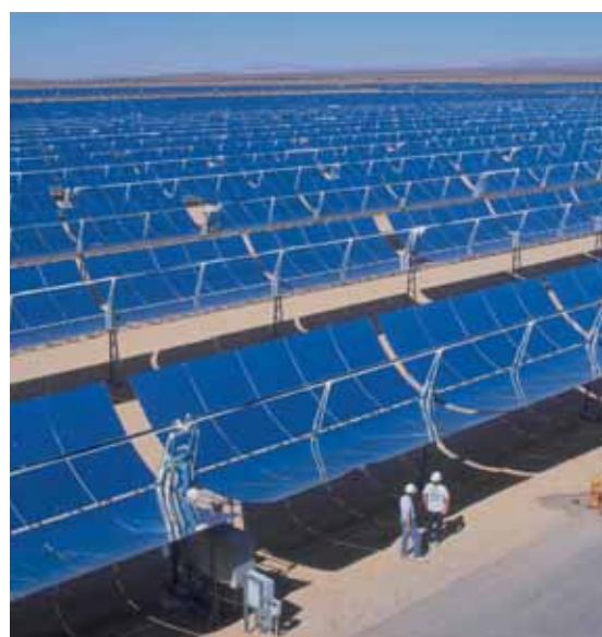
A concentrating solar power plant located at Kramer Junction in the Mojave Desert, California, USA.
