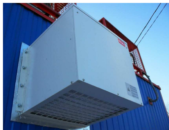
Stulz free-cooling system
