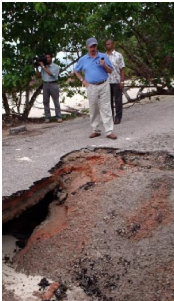
Mahé Island, Seychelles (27 December 2004). President James Michel of the Seychelles inspects damage to infrastructure in the Seychelles. Initial assessments of damage to roads, fishing infrastructure, agriculture, public utilities, schools, land, houses, sports facilities and tourism establishments indicated damage amounting to $30 million. © George Thande/Reuters
